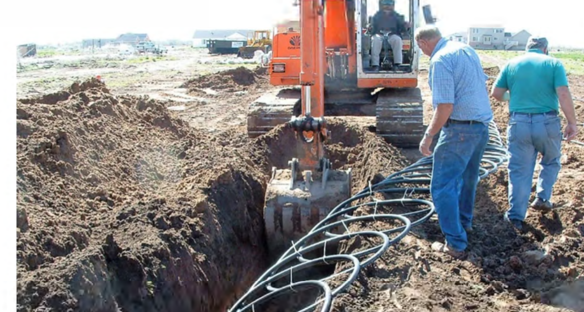
Figure 2: HDPE loop in slinky configuration being dropped into a trench. [Courtesy Centennial Plastics]
