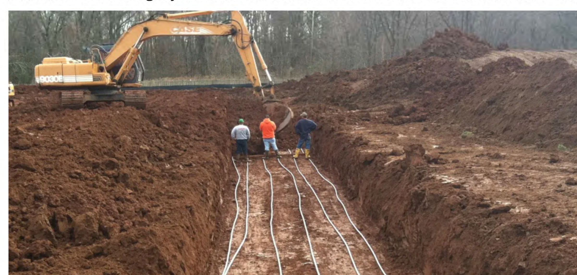
Figure 3: PEX tubing used as horizontal ground loops
